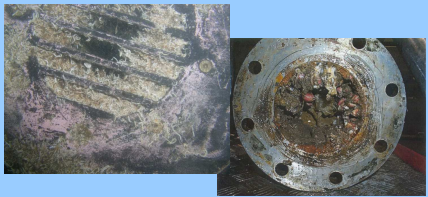
Poorly Protected Internal Seawater Systems (Defence)
